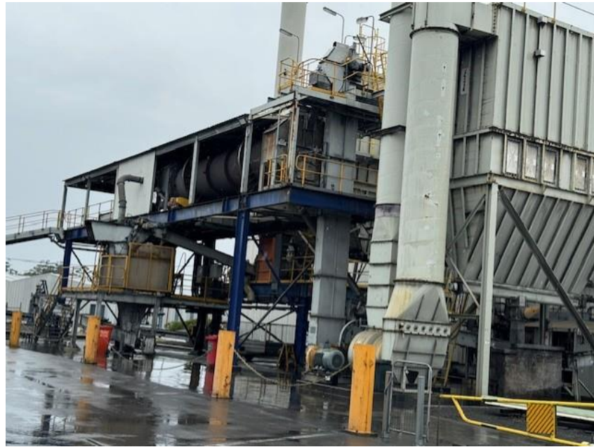
Photo 9 – Thermal Treatment Plant No 2 Dust Collector
