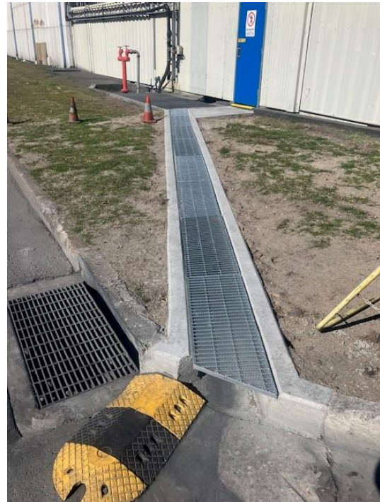
Photo 8 – Stormwater Interception Drain
