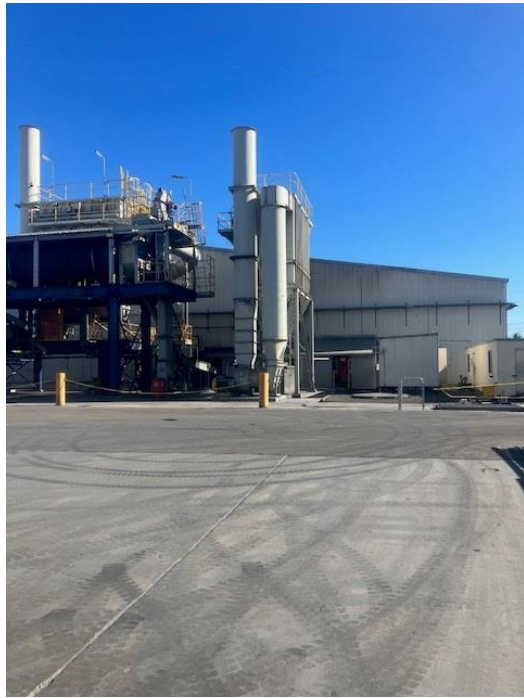
Photo 9 – Thermal Treatment Plant No 2 Dust Collector
