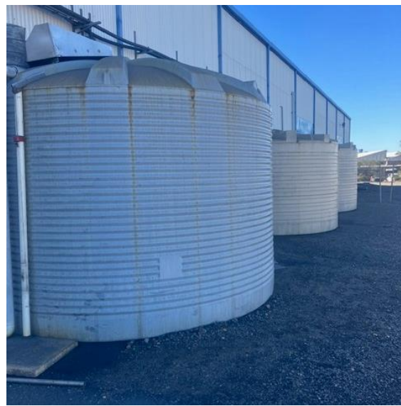
Photo 6 – Stormwater Storage Tanks
