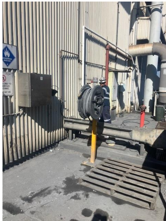
Photo 7 – Washdown Water Hose
